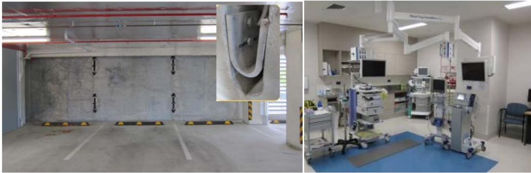
Figure 2-6. Negligible observed damage to the Southern Cross Hospital designed with a rocking-dissipative solution during the Christchurch earthquake (Pampanin et al. 2011)
